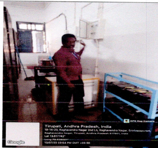
POWER BACK UP SYSTEM ON COLLEGE OFFICE PREMISES
